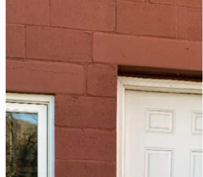
Horizontal cracking at pre-cast lintel and along vertical mortar joints
