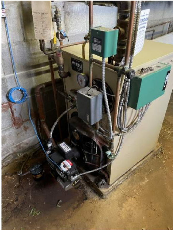
Oil Fired Boiler
