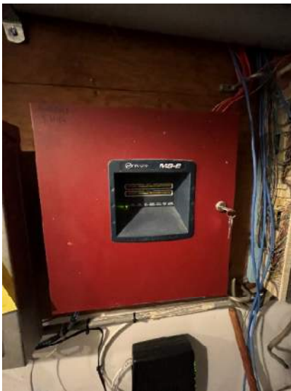
Fire Alarm Control Panel
