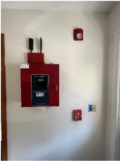
Fire Alarm Control Panel
