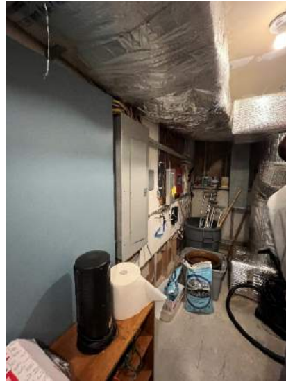
Main electrical panel
