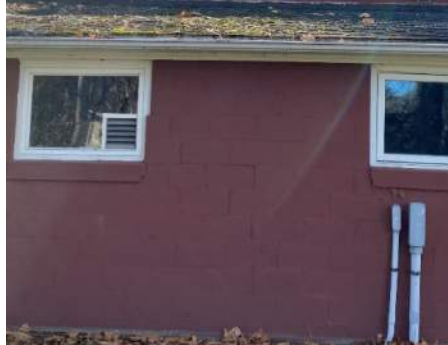
East Elevation – mortar joint crack
