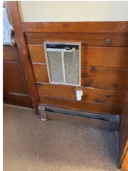
Wall heater and baseboard heater at entrance
