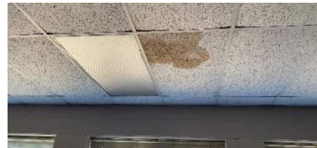
Water stains at classroom ceiling
