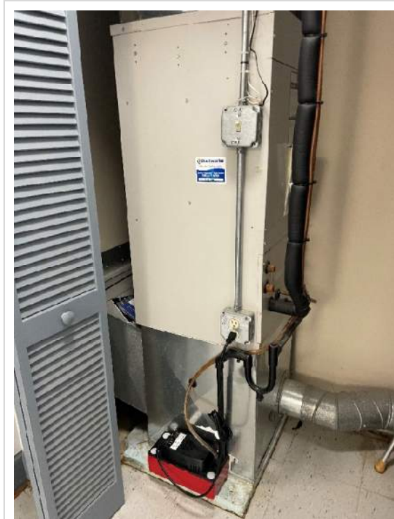
Typical Vertical AHU on Lower Level
