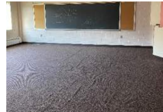
Wrinkled carpet in classroom
