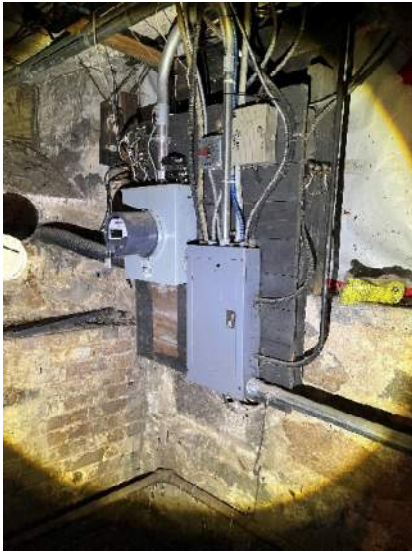
Main Electrical Service Equipment
