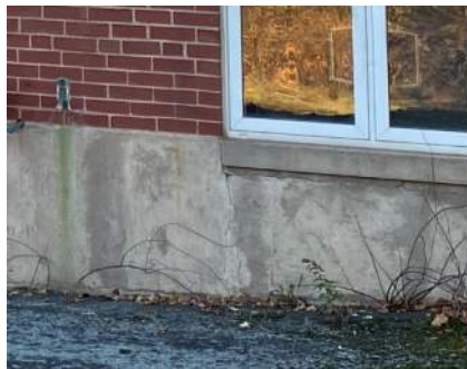
Crack in cast-in-place foundation
