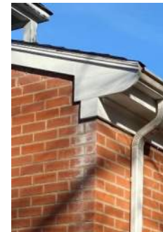
Staining on brick
