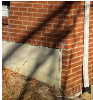
Cracking at concrete foundation joint near brick
