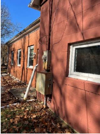
Electric service entrance and meter
