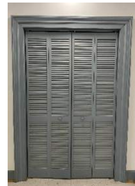
Mechanical closet door
