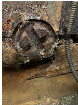
(2) Corrosion at bottom of boiler #1
