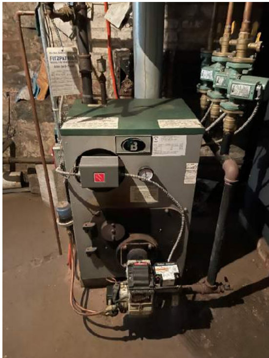
Hot Water Boiler
