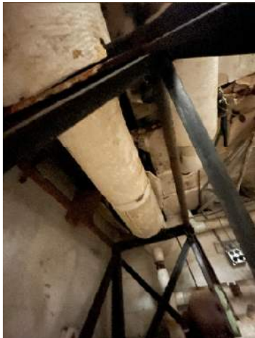
Shell and tube steam to hot water heat exchanger
