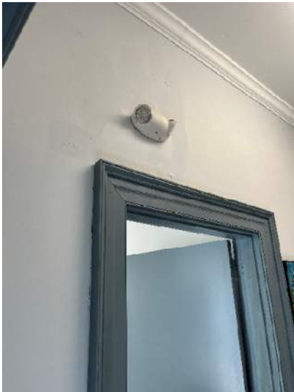
Self-contained emergency light
