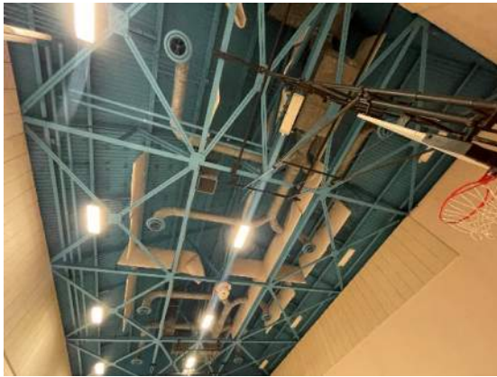
Air Handling Units at Gym
