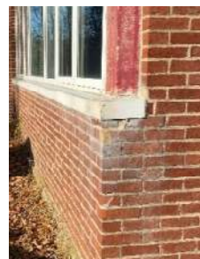
Staining, cracked brick
