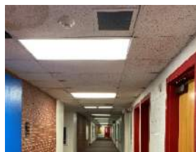
Water stains, corridor
