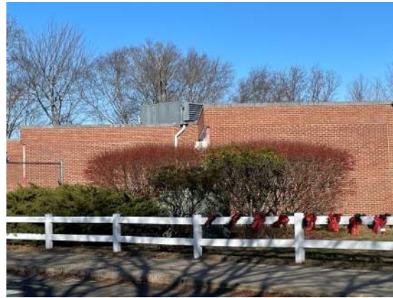
AHU with energy recovery on roof of West Wing
