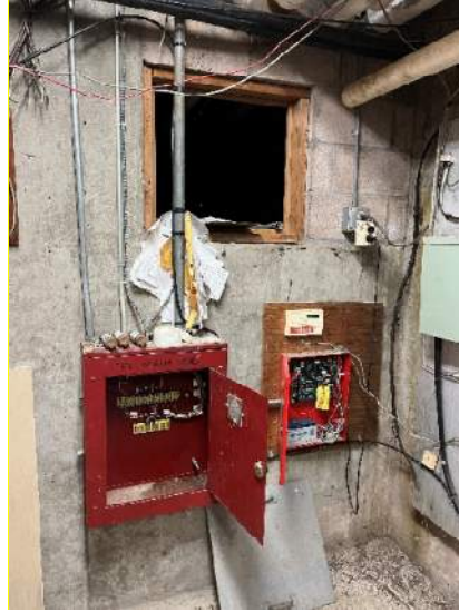
Fire Alarm Control Panel and Splice Box
