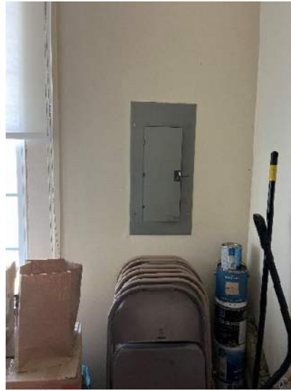
Main Electrical Panel
