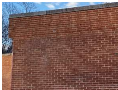
Open mortar joints and spalled brick & column requiring painting
