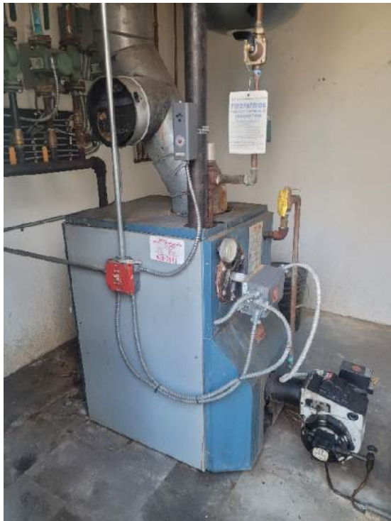
Oil Fired Boiler
