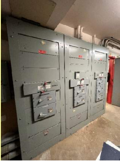
Main Electrical Distribution Equipment
