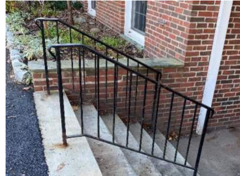
Staining on masonry
