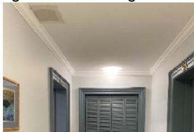
Basement corridor ceiling with water stains
