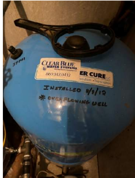
20-Gallon Well Storage Tank
