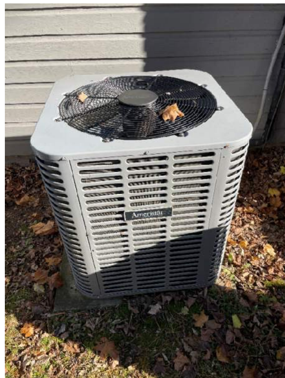
Grade mounted Condensing Unit
