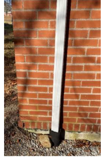
Discharge to underground piping
