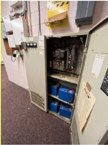
Central emergency lighting inverter
