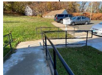
Efflorescence and cracking at bottom of ramp
