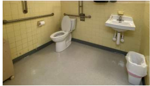
1 st Floor VCT in toilet room
