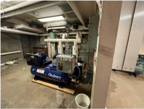
Compressor for pneumatic controls
