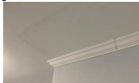
Cracking corridor ceiling
