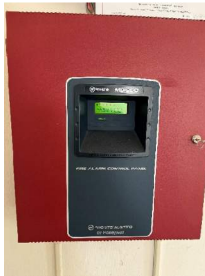
Fire Alarm Control Panel
