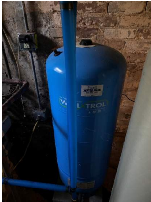
Well Storage Tank
