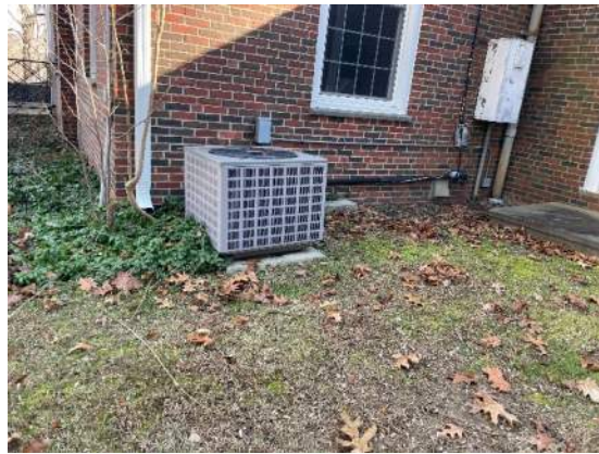
Condensing unit located on grade
