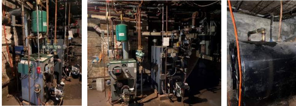
Mechanical equipment in basement
