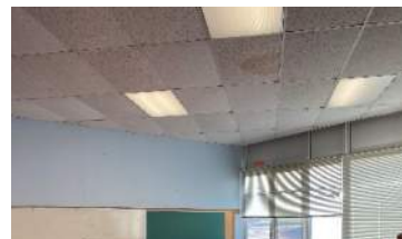
Water stains and sagging
