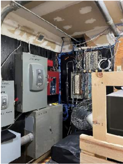
Main electrical service equipment
