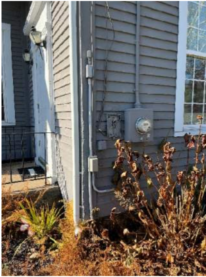
Electrical service entrance and meter
