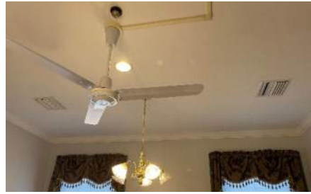
Ceiling fan and lights
