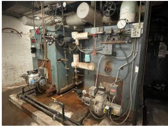
(2) Oil Fire Steam Boilers
