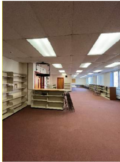
Typical 2'x4' lighting
