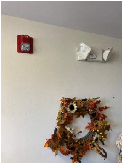
Self-contained emergency light and strobe
