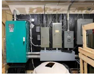
Basement electrical panels
