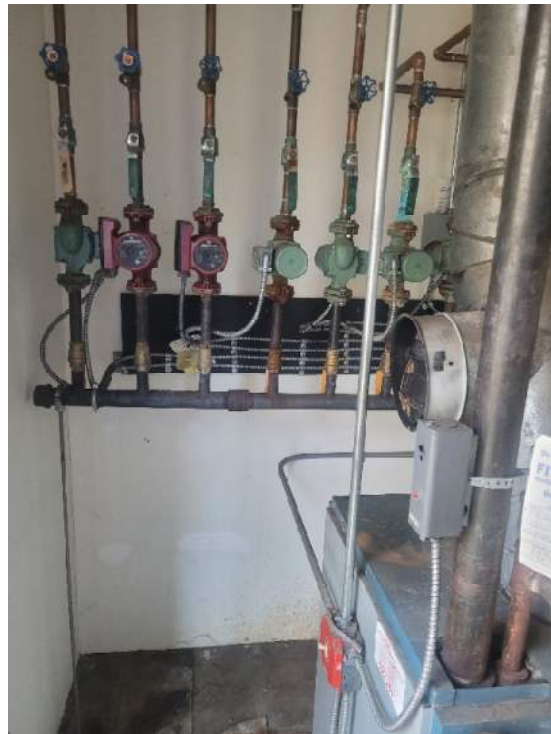
Heating Hot Water Zone Pumps
