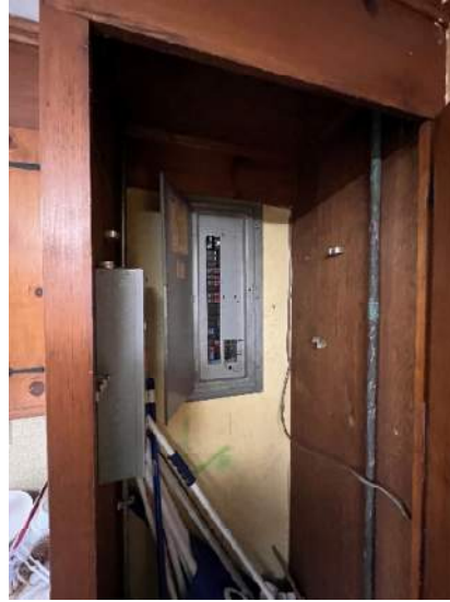
Main electrical panel
