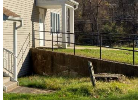
Cast-in-place retaining wall, areas of cracking and spalling
