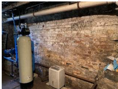
Masonry foundation. Visible efflorescence
