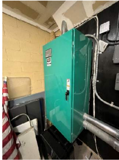
Automatic Transfer Switch (ATS)
