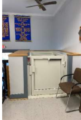
Lift at 1 st Floor
