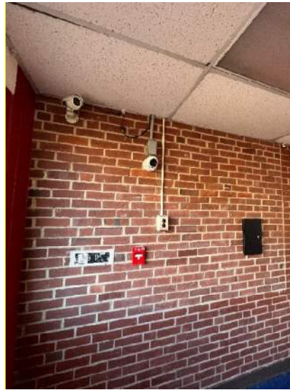
Main Entrance Lobby equipment
