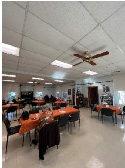
Typical 2'x4' lighting
