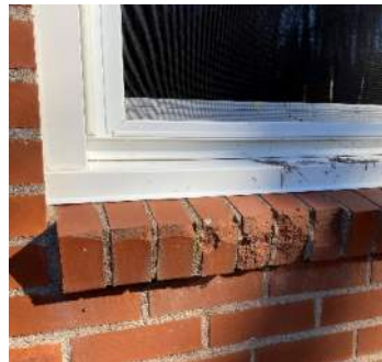
Damaged brick at window sill
