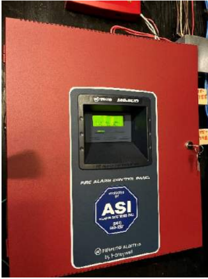
Fire Alarm Control Panel
