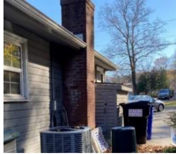
Visible efflorescence at chimney
