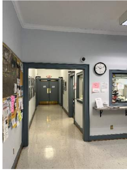
Main Lobby video surveillance camera
