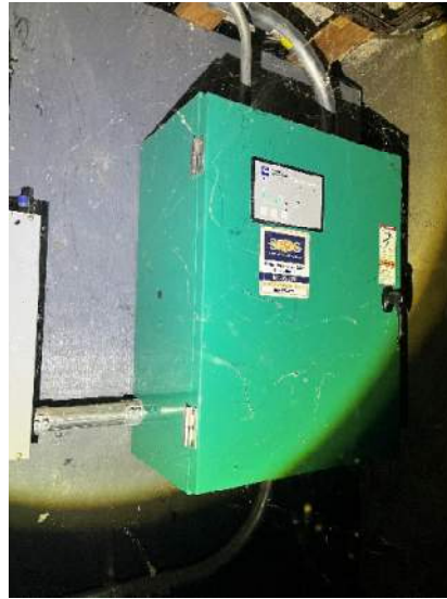
Automatic Transfer Switch
