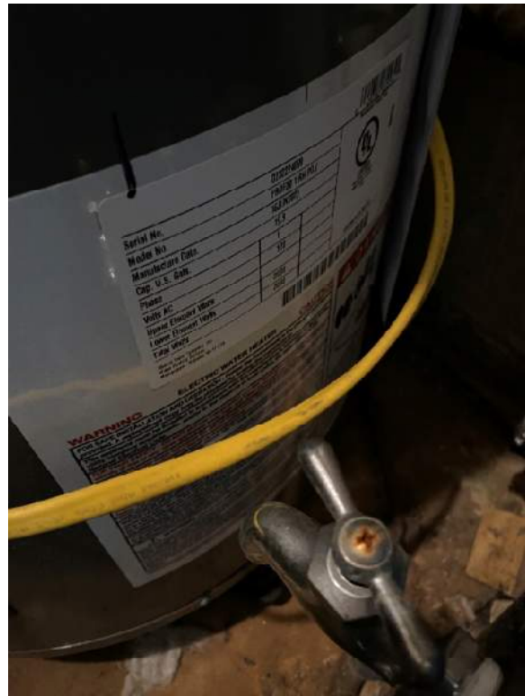
Water Heater Manufacturer Plate
