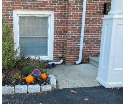
Cracking at masonry near down spout
