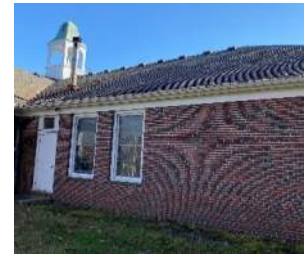
Moss on roof
