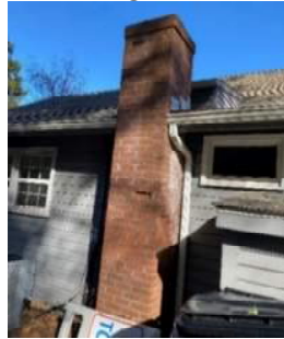
Spalled masonry at chimney
