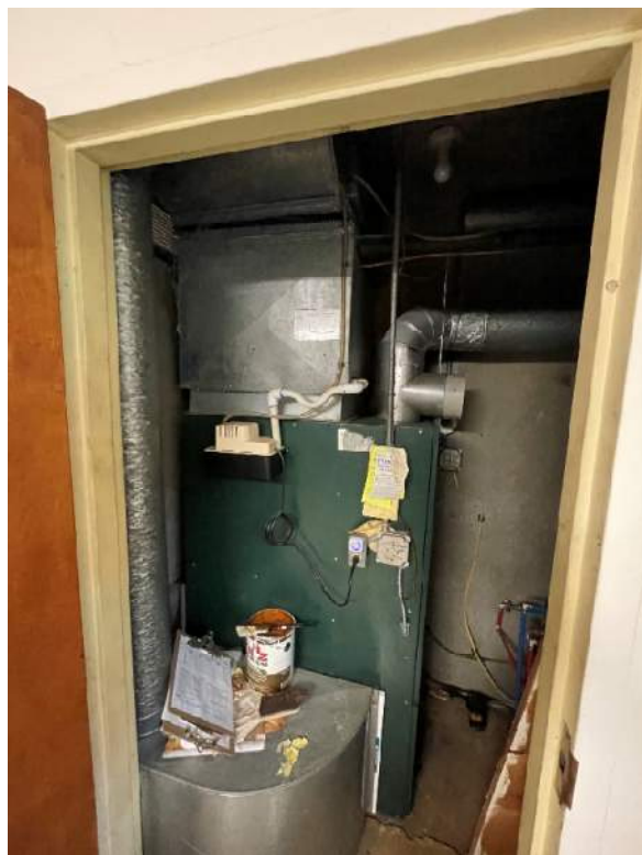
Vertical Air Handling Unit
