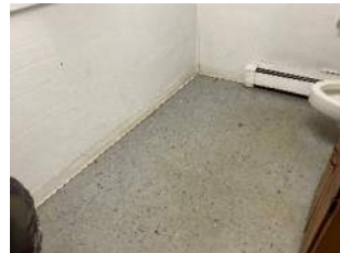
VCT in toilet room
