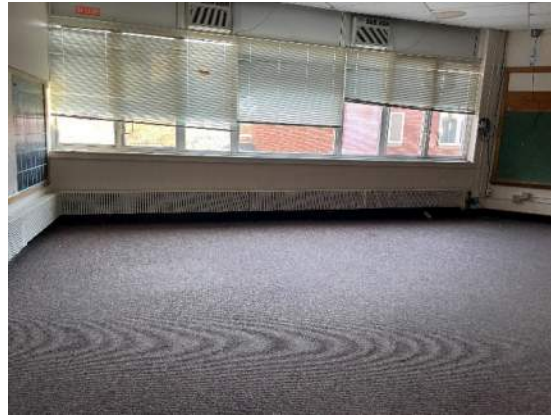
Classroom with perimeter radiator and (2) through wall air conditioning units
