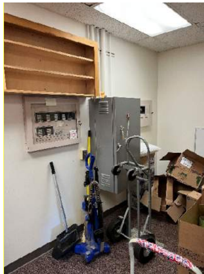
PA System headend equipment
