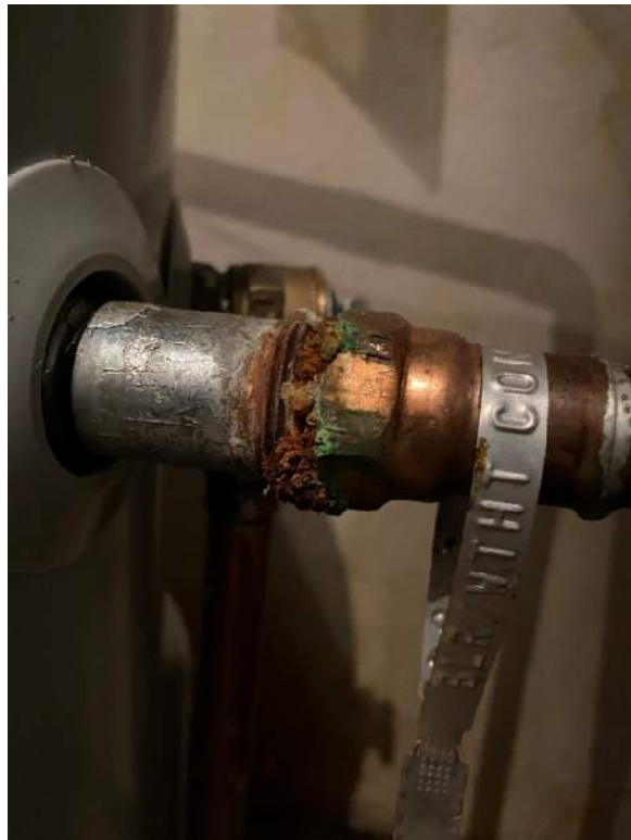
Water Heater Outlet Connection
