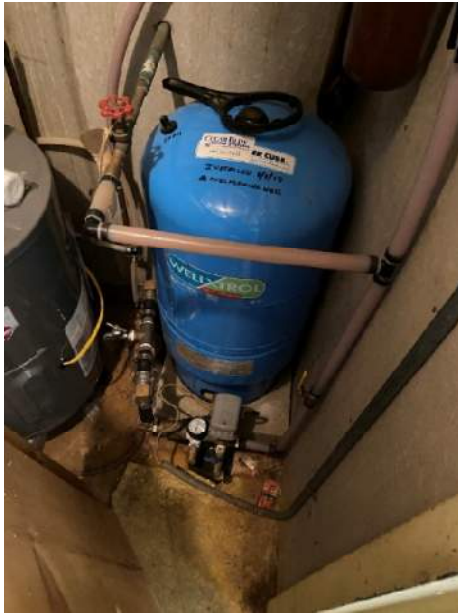
20-Gallon Well Storage Tank
