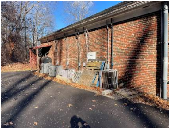
(5) Condensing unit located on Grade at back of building
