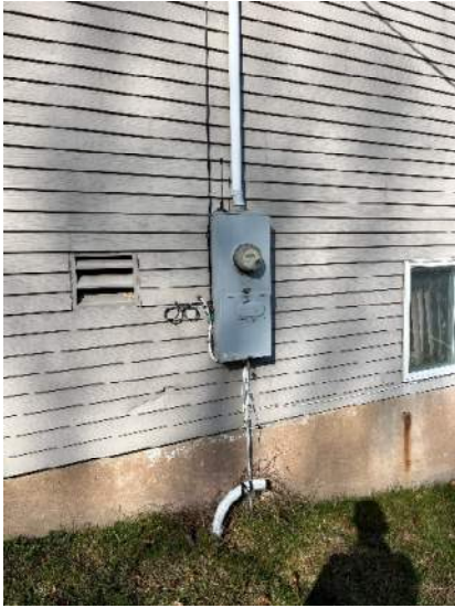
Electric service entrance and meter
