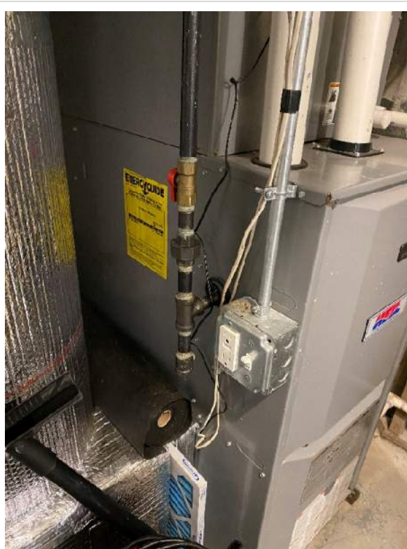
Propane Gas Piping to HVAC Unit
